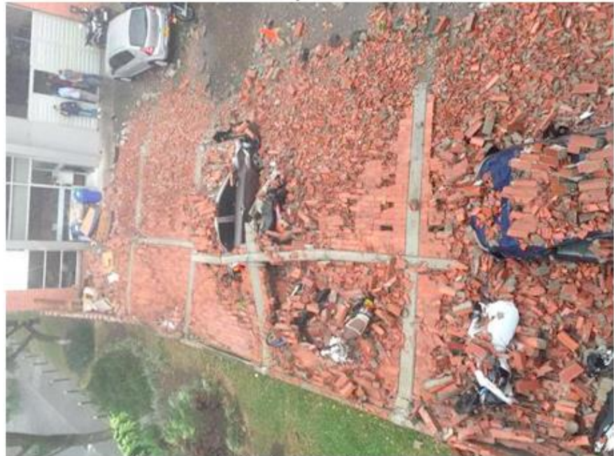
(b) Muro colapsado
